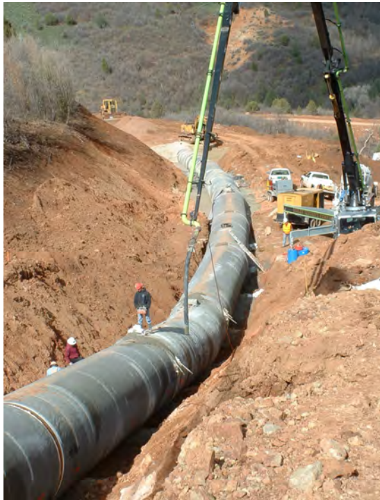
Diamond Fork Pipeline
