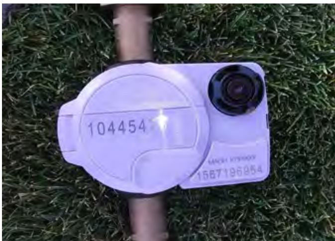
A meter for secondary water.
