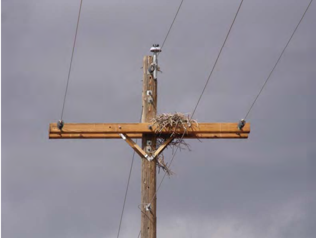
Figure 7 Nest structure on power pole 3 miles south of Cedar City
